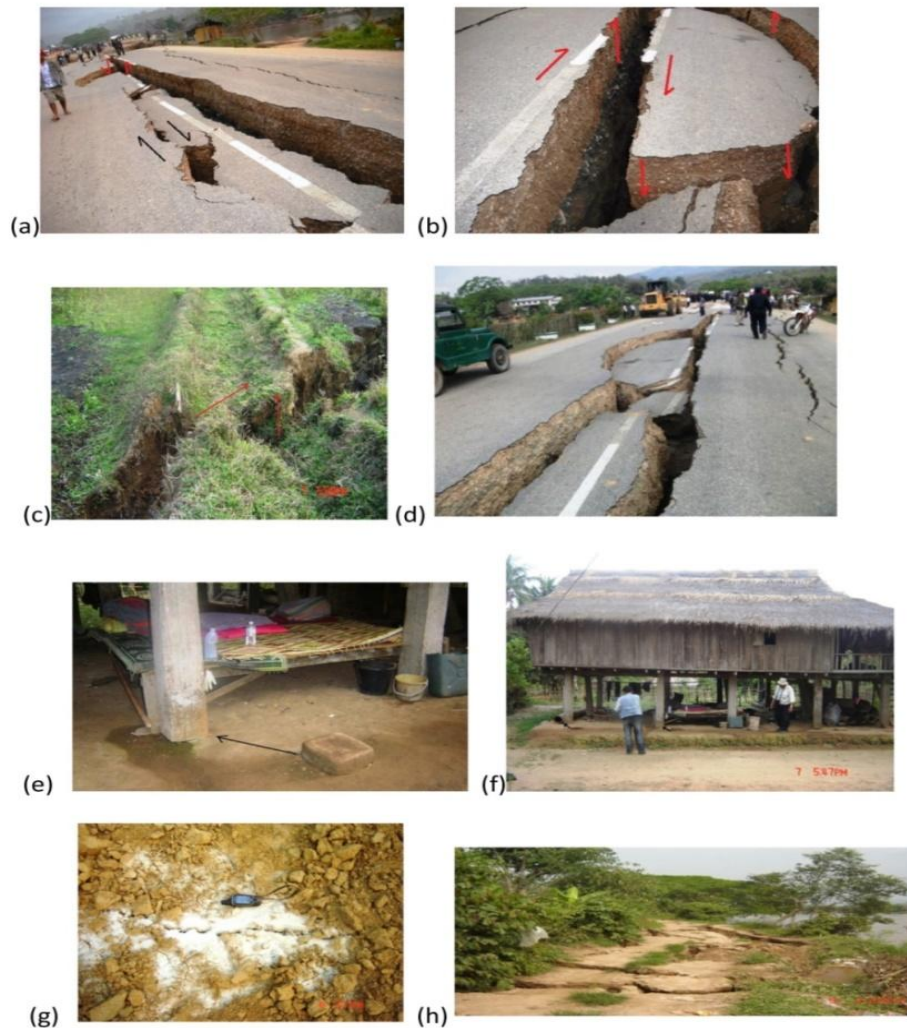
Fig. 2. Photographs of surface deformation produced by the Tarlay earthquake along the rupture zone. (a,b,d) The ground crevices split and settle down like rifting on the road. (c) The ground crevices split and settle down like rifting in the paddy field. (e,f) columnar of the house shifted due to lateral displacement by the earthquake. (g) Sand extrusion as liquefaction features. (h) Ground fissure system in the village near Tarlay town
